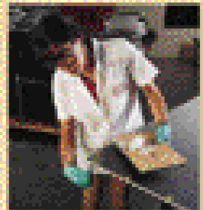
Technician smoothens the edge fill compound and ensures there are no air bubbles along the panel's edges.
