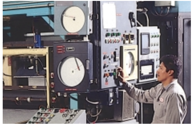
2. The master control panel regulates print roller and cutter, paper humidity, and printing oven in the processing that follows.
