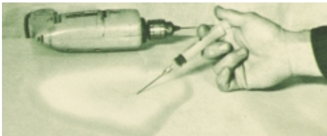
Blister delamination—using a 10cc syringe, inject blister with thin epoxy adhesive. Apply pressure until adhesive cures.
