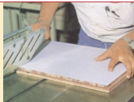
This panel is being cut on a table saw using a diamond grit blade with a backing piece (in this case, plywood) under the panel.
