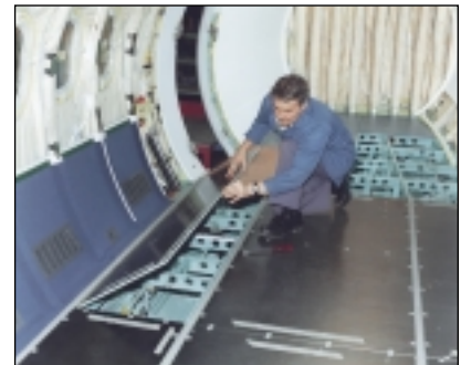
British Aerospace employee installing carbon faced/Nomex honeycomb flooring in the BAe 146 passenger area.
