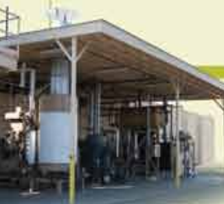
Low-NOx boiler system.
